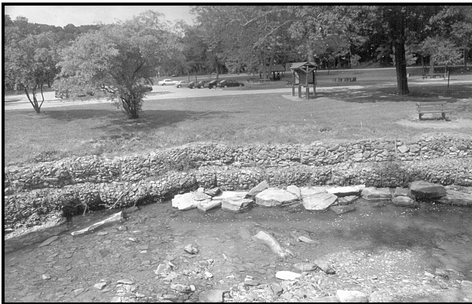
Stormwater impacts: Many sections of Euclid Creek have been eroded and damaged from flood waters tearing downstream during rainstorms. Here stone gabions have been installed to reinforce the stream bank.
